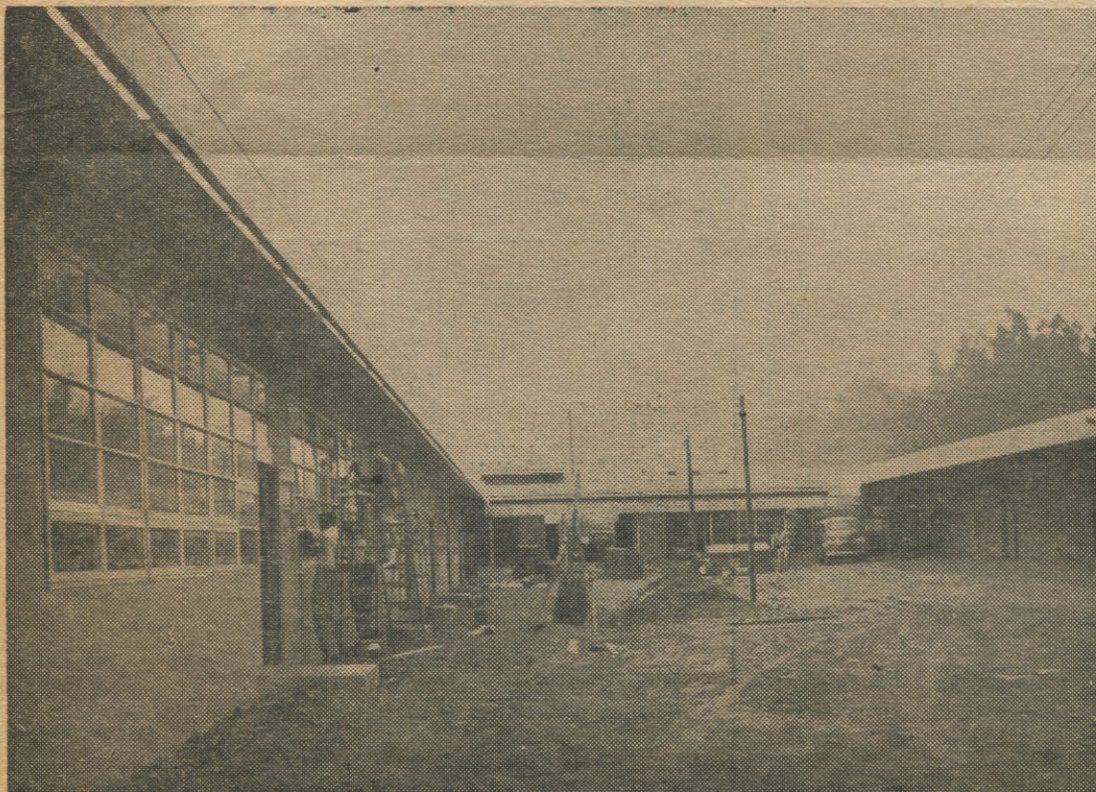
Workmen are busy putting on the finishing touches on the classroom buildings so they will be ready for completion November 2.
